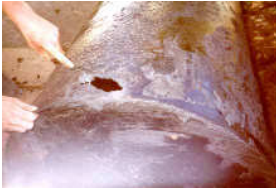
Hole in Underground Storage Tank found after removal
